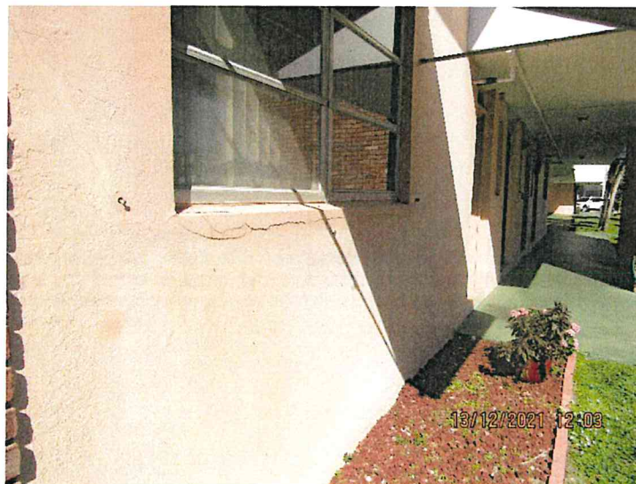
4. View of crack in concrete wall below window sill. Please repair.
