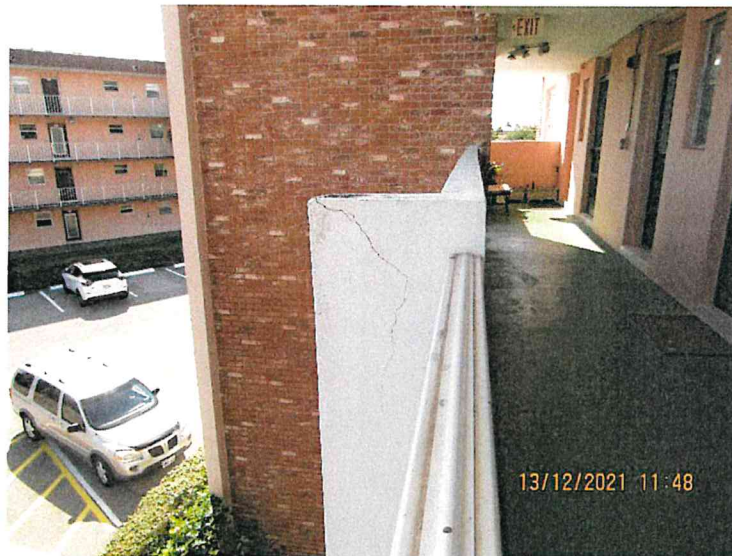
3. View of crack in concrete wall of 3 rd floor balcony. Please repair
